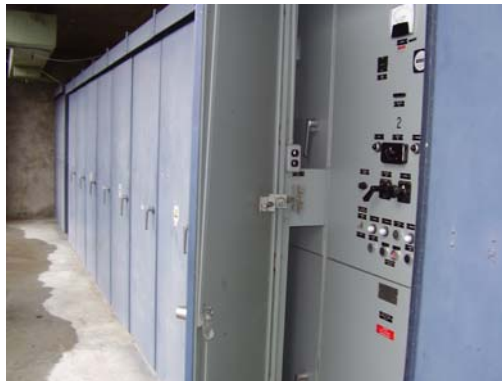
Motor Control Center
