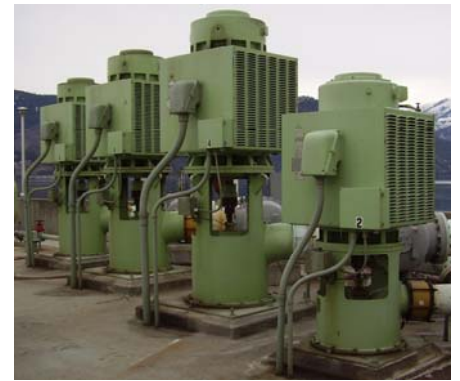
Pumps And Motors
